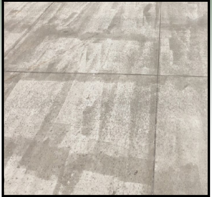
UNEVEN APPLICATION OF SEALER WITH ROLLER
