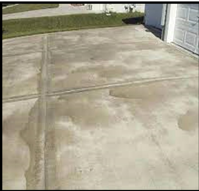
OVER APPLICATION OF SEALER
